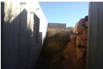
Concrete stairs needed
